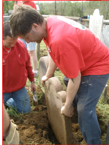
Left: sandstone being reset. Note the marks showing where the stone was buried with only the top showing.
